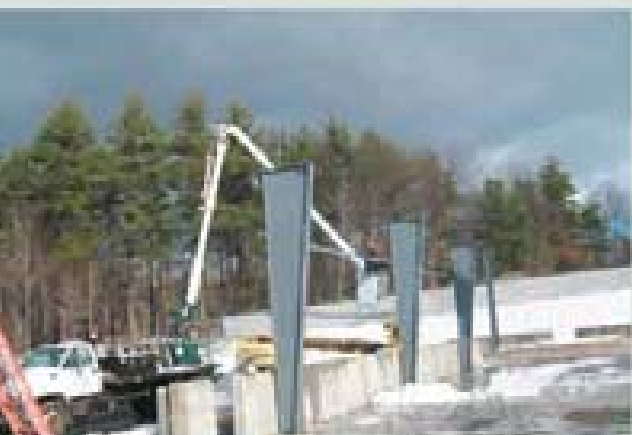
Girts are attached to tapered column sections of rigid frame as assembly of Butler Building begins.
