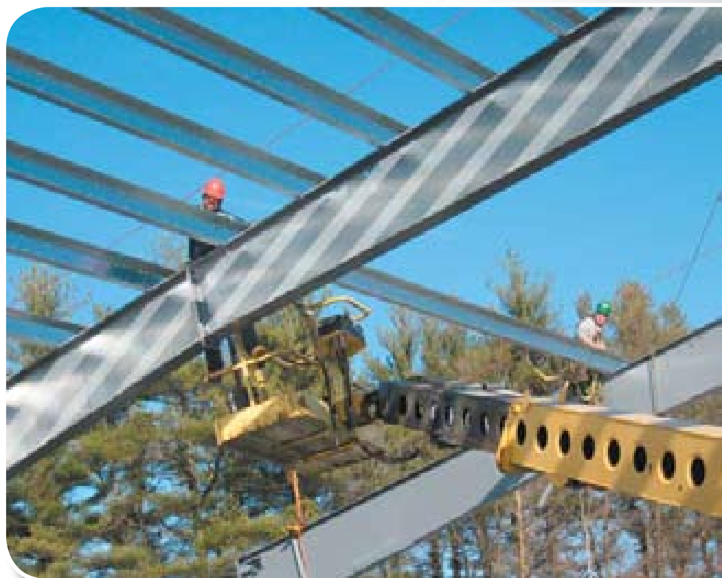
Raymond Brothers worker on a Grove lift attaches roof purlin to frame of Butler Building being built by Maple-Leaf Construction in Hudson, N.H.
