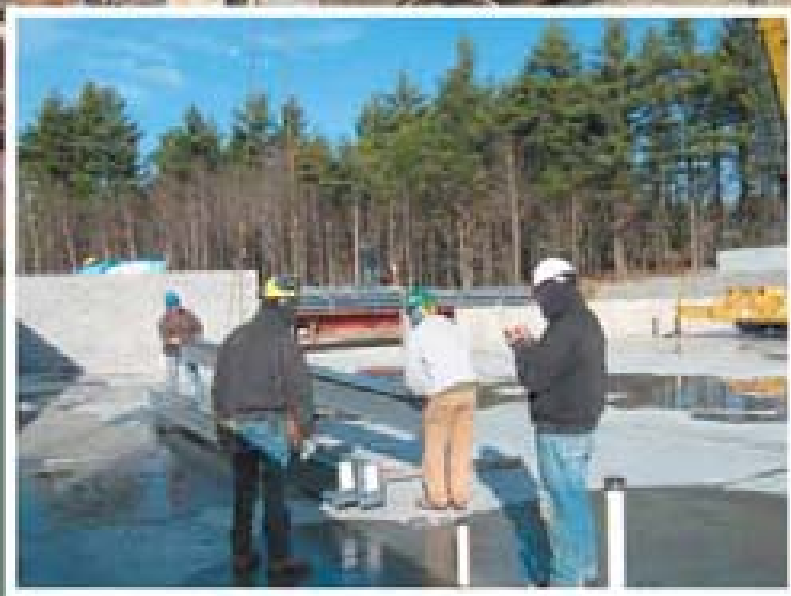
Maple-Leaf Construction job superintendent Mike Marois, at right, checks master list as coded building components are delivered.
