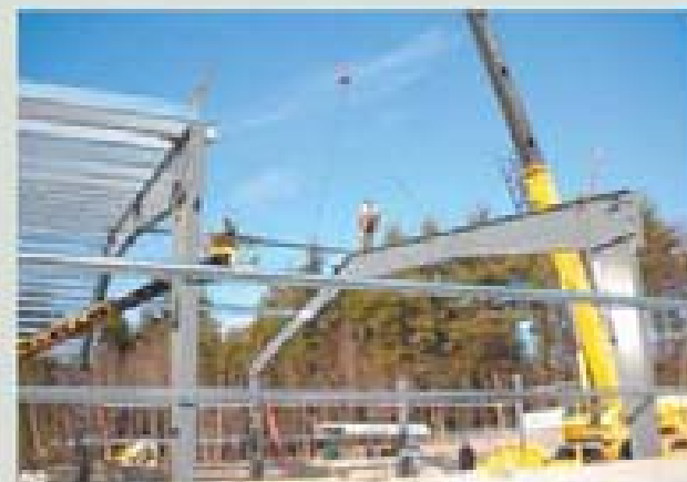
Crane holds rigid frame in place as workers tie frames together with roof purlins.
