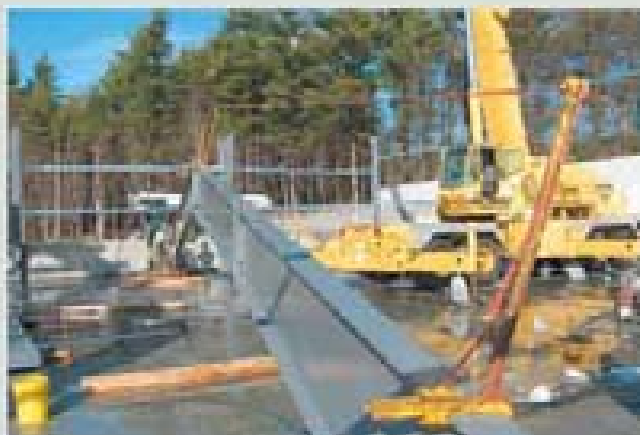
Roof beam sections of rigid frame are put together as Grove crane gets ready for lift to top of columns.
