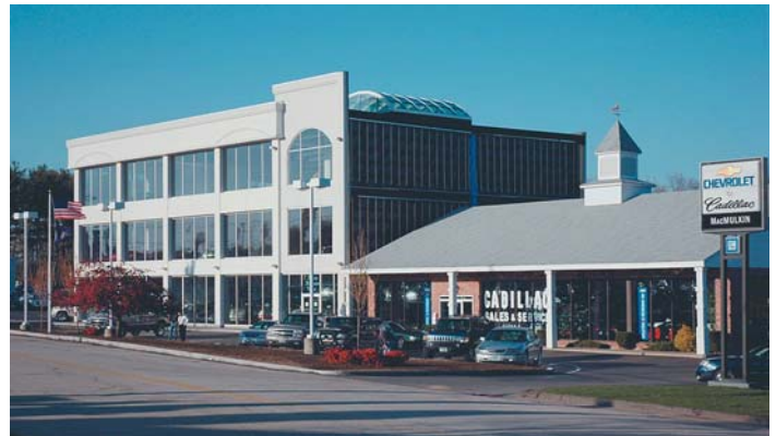
A view of the completed Phase II, showing temporary sidewall and existing showroom. Upon the completion of the move into the new showroom, the existing single-story showroom will be demolished, and the Phase III wing added to complete the project.
